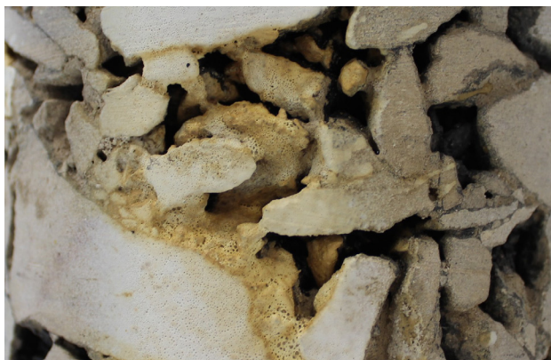
*Image shows contaminated tar
